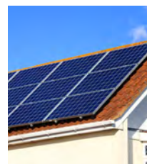
Domestic Solar Panels
